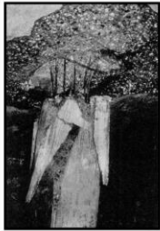
Port of Oakland, 1989 Loma Prieta Earthquake
